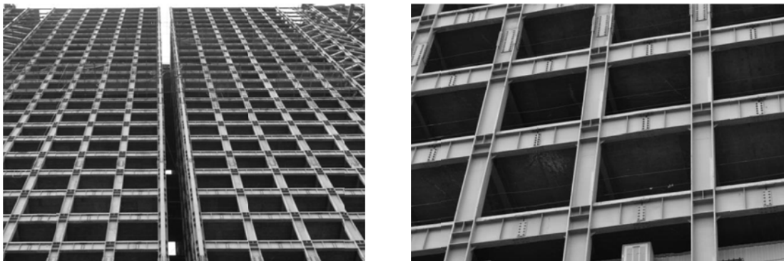
Figure 2. 34-story framed tube structure with beam splices at the mid-span of the beams; Third Millennium Tower (TMTower), Tehran, Iran (Photos by M.T.Nikoukalam).
